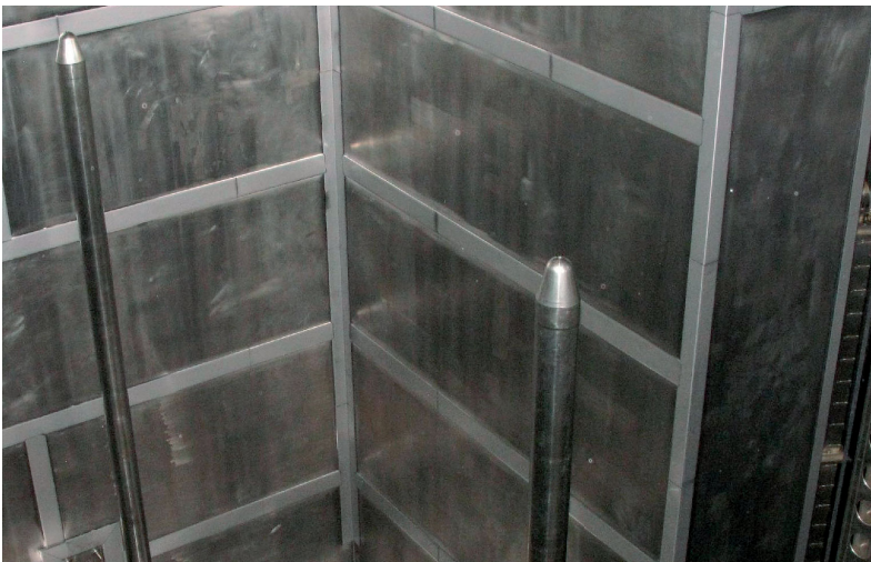
Reactor cavity repair: all welded joints were covered as a preventive measure
