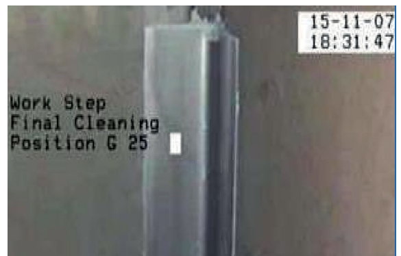
Remotely repaired SFP corner
