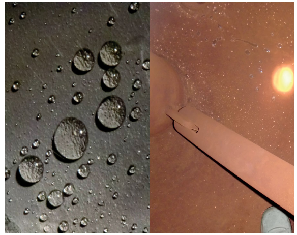
Visual inspection and water droplet test: condenser floor and protected oxide layer
