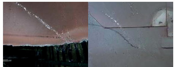
Visual inspection and water droplet test at a PHWR: cut feedwater line (raw edge), moisture separator inside (welded area)
