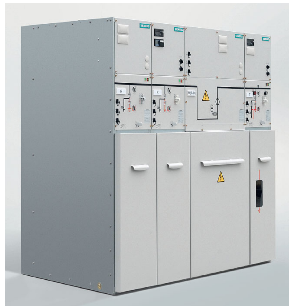
Medium Voltage Feeder
