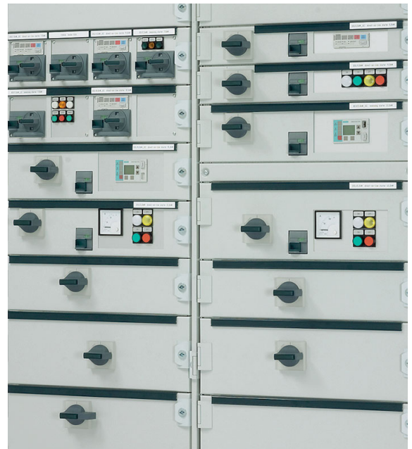
Low Voltage Feeder
