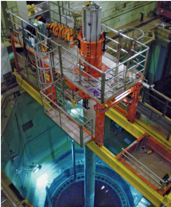
Installed CMM system
