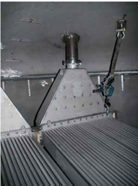
Containment Cooling Condenser
