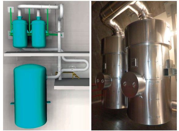
Example of an installed retrofit solution
