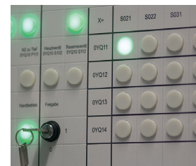
Manual Control Station
