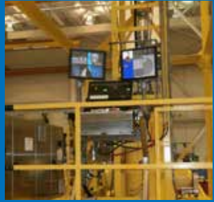
Stearns Roger Automated Refueling Bridge
