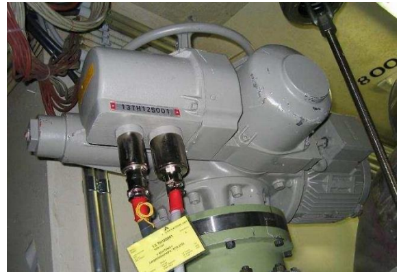
Motor-operated valve being reassessed
