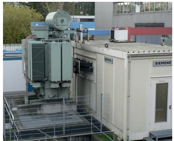
Karlstein High-Current Source: power supply with rectifier
