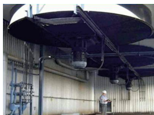
25 MW high pressure heat removal system
