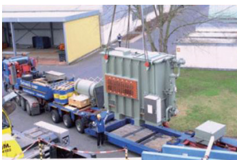
New transformer for 20 MW grid connection
