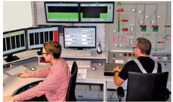
KATHY control room
