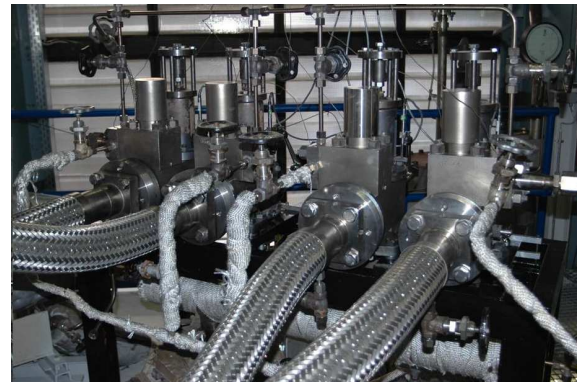
Test set-up for hot adjustment of pilot valves on the valve test array
