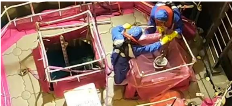
Massive TC replacement performed on a floating platform with TC continuous insertion tool
