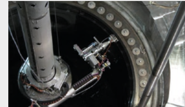
Primary circuit components PSI* and ISI* at nuclear power plants
