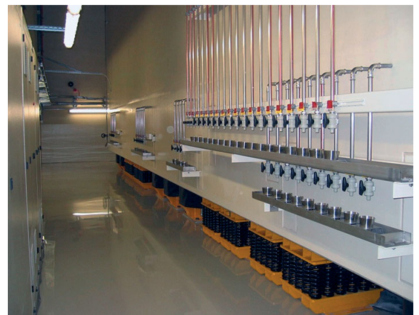
Seismic isolation supporting the spent fuel pool structure
