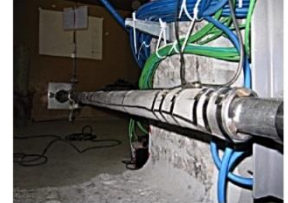
Double wall pipe in room without leak retention
