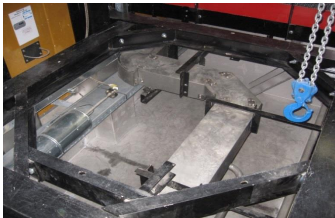
Drainage area in TND before fitting a tank. View of the supports and retention trays
