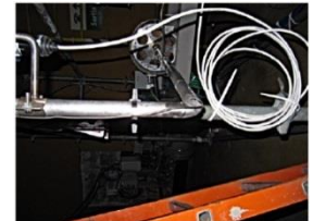
Drainage line section connected to an electromagnetic pump
